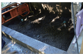
The filter tank is filled with fine gravel.
