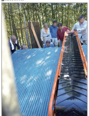
Place the belt conveyor on top of the filter tank with the lid closed, and the work is complete.
