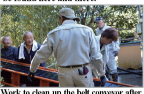
Work to clean up the belt conveyor after washing the gravel. A smile spills over my face after completing nine minutes of hard labor:
