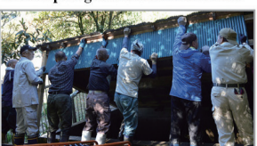
Finally, close the filter tank lid. It's heavy so we'll all have to tackle it together:
