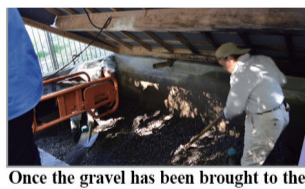
Once the gravel has been brought to the washing area, it is unloaded from the belt conveyor to the washing area.
